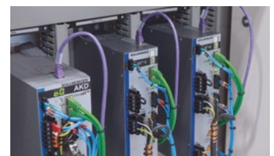
EtherCAT control system
